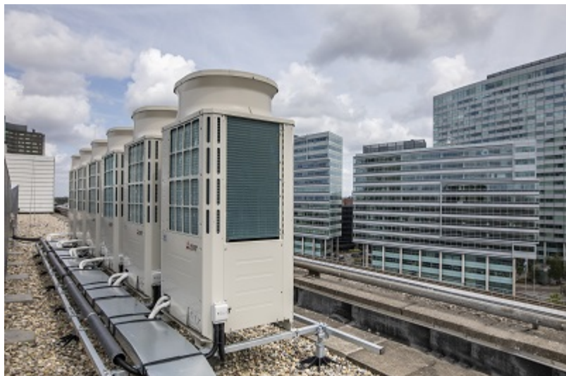
City Multi VRF R2-buitendelen van Alklima/Mitsubishi Electric.
